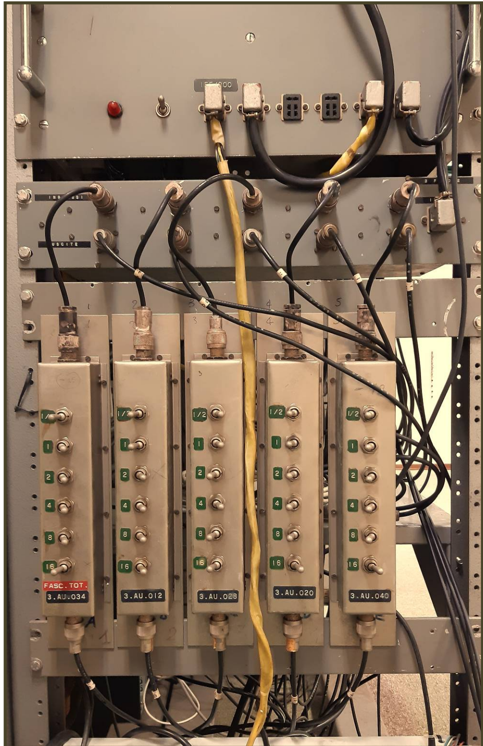
Rivelatori Fasci NS – Rack 29
