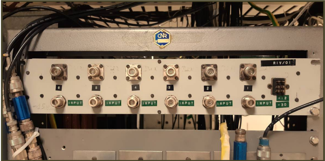
Rivelatori Ch EW – Rack 21
