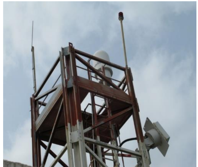
Figure 2. The “Flight Termination System” (FTS) transmitter
