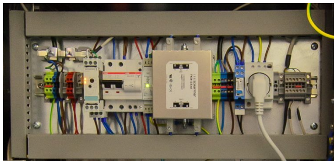
Figure 6 Electrical components in the FEU cabinets
