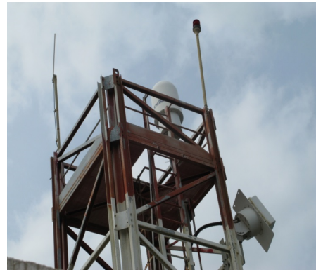
Fig. 1. The "Flight Termination System" (FTS) transmitter.
